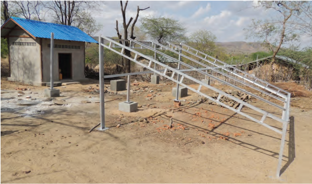
Mounting rack for photovoltaic panels during mini-grid installation
