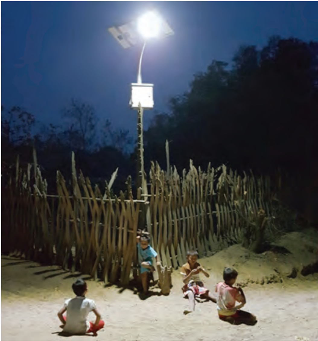
Streetlight in one of the pilot projects
