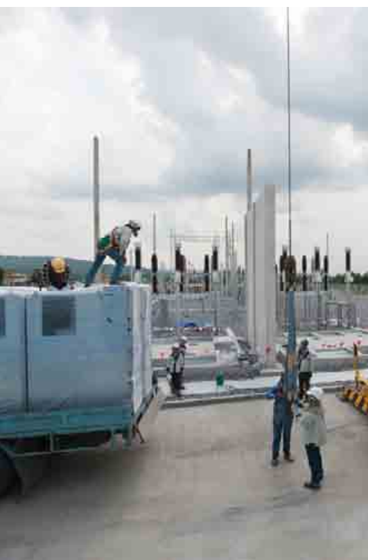
■ Upper and Lower: Construction of the Lop Buri solar power project, Thailand.
