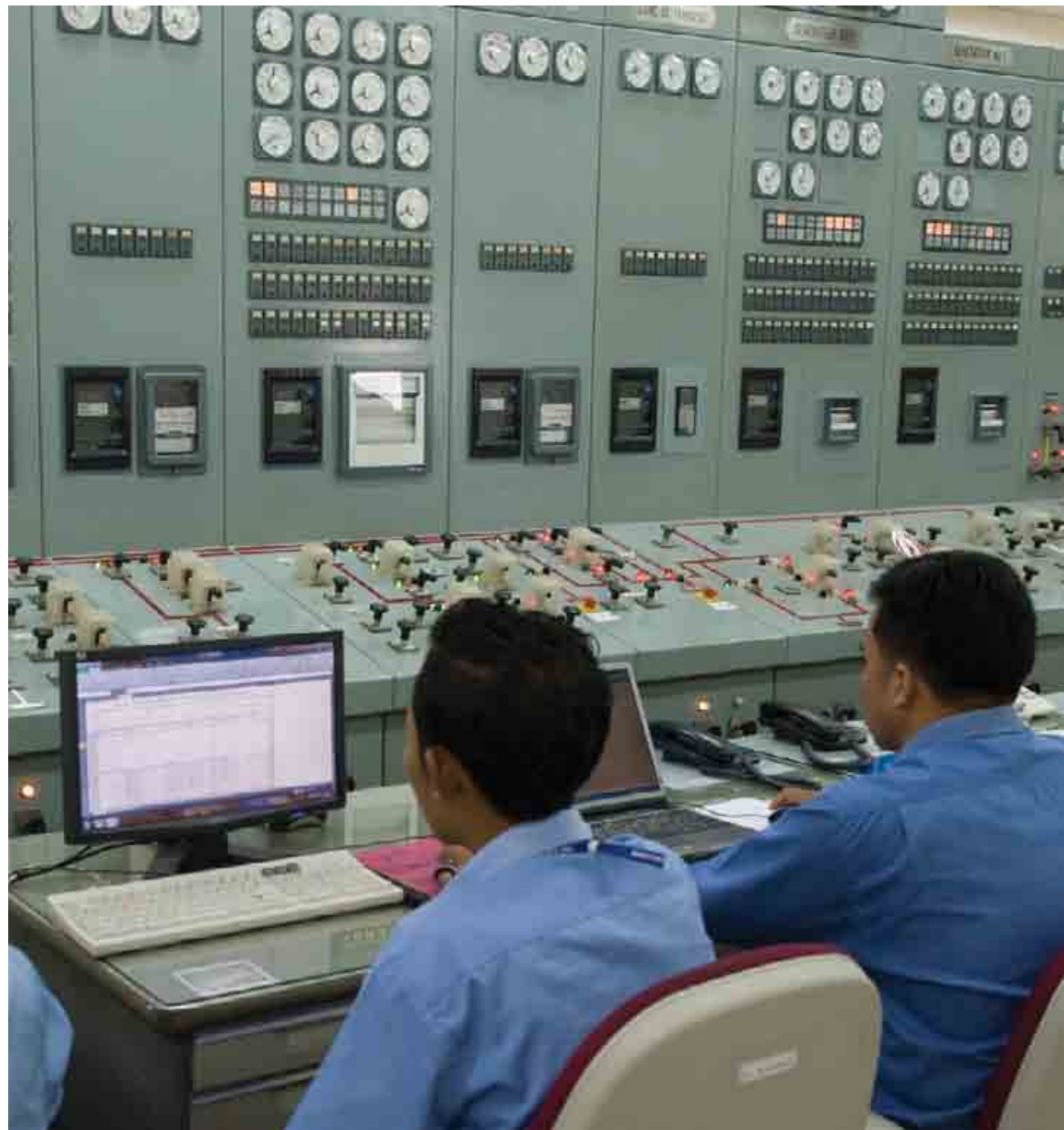
■ Control room of the Nam Ngum 1 hydropower plant, Lao PDR.
