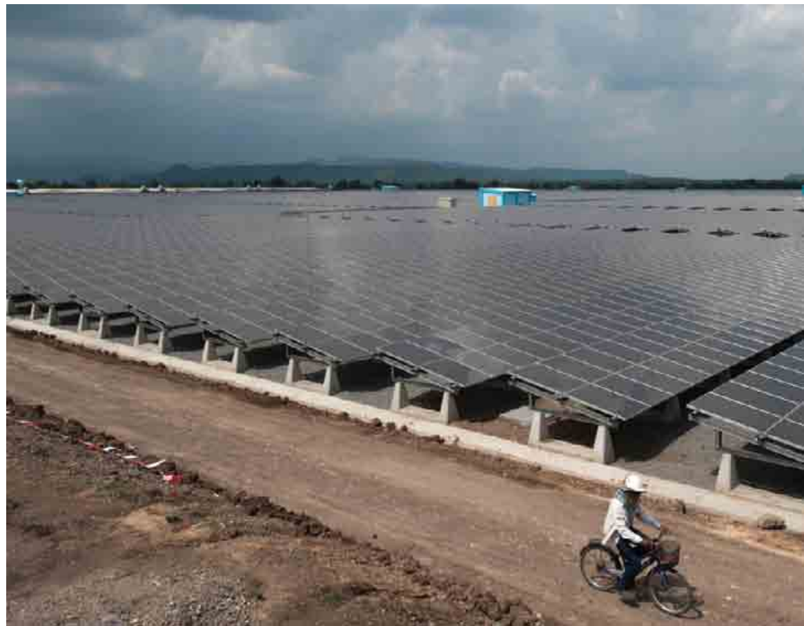
■ Solar panel array of the Lop Buri solar energy project, Thailand.
