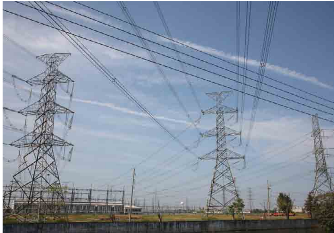
■ Power transmission lines, Thailand.
