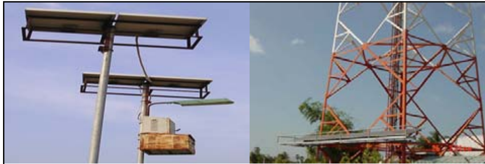
Solar PV for Bridge Lighting and Telecommunication Systems
