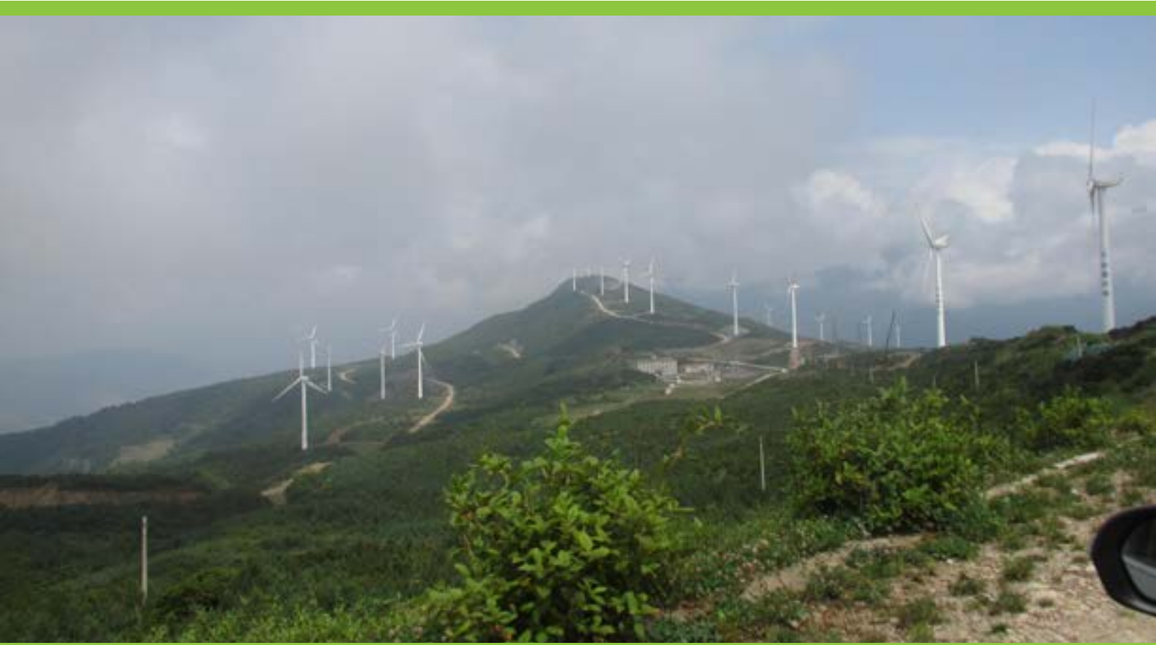
Zemoshan wind farm with 61 windmills with 45.75 MW capacity, Daly, Yunnan, People's Republic of China
